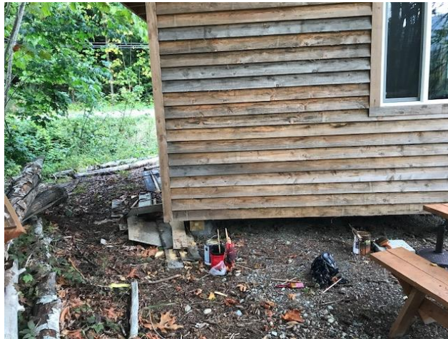
Various combustibles within Zone 1a 1.5 m around home
